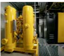
Compressed air systems: dryer monitoring to avoid damage caused by humidity
